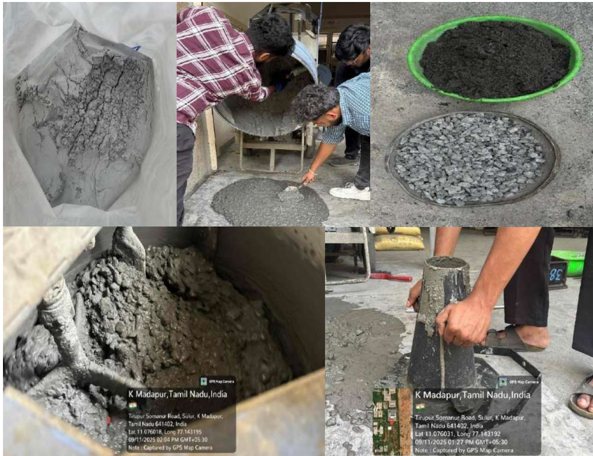
Fig 5.1 Concrete specimen Batching and Mixing Procedure
